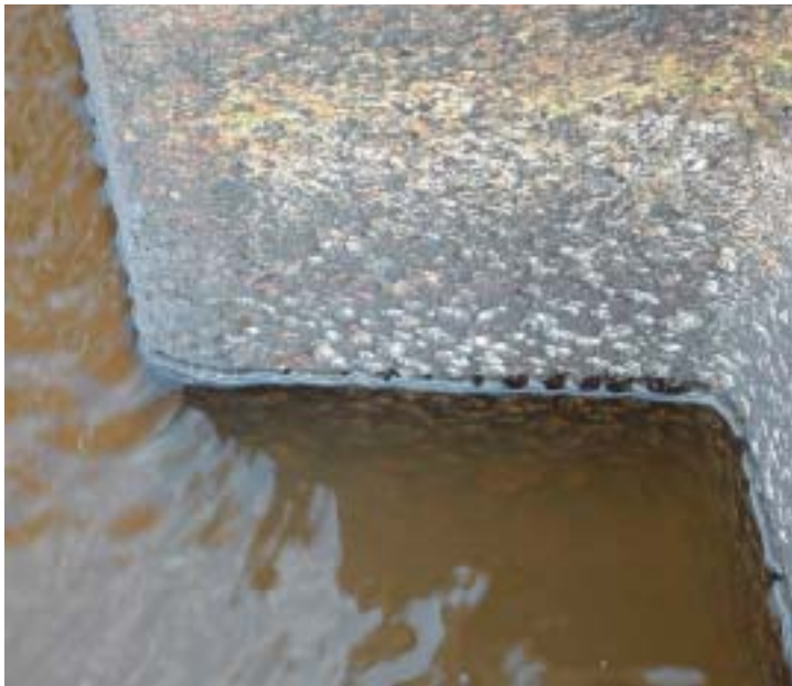
Researchers examined 12 possible causes of the accelerated corrosion; the exact cause still remains a mystery.
