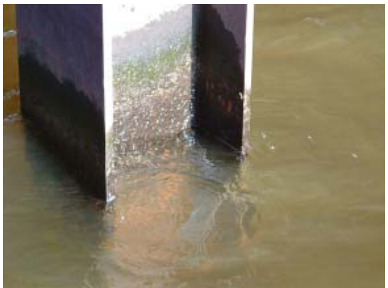
Most of the corroding steel sheet pilings and beams—which may require up to $100 million to repair—are riddled with pits.
