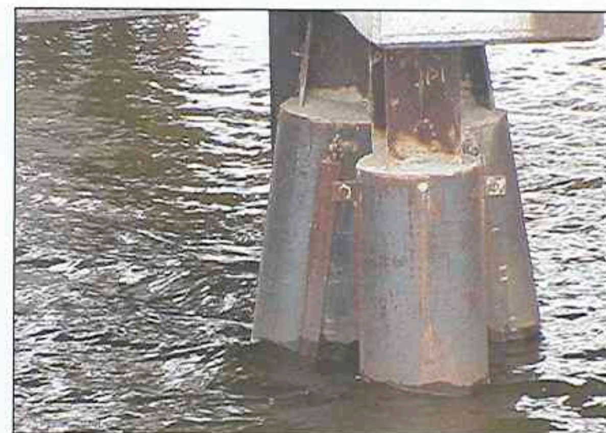
You can protect "H" piles by putting a jacket around them and filling with concrete, but this is not very practical for sheet piles.
