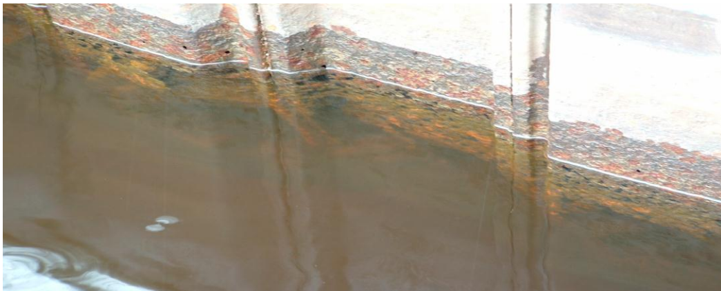
Photo 2. Sheet Pile Pitting and Large Perforations at Local Marina
