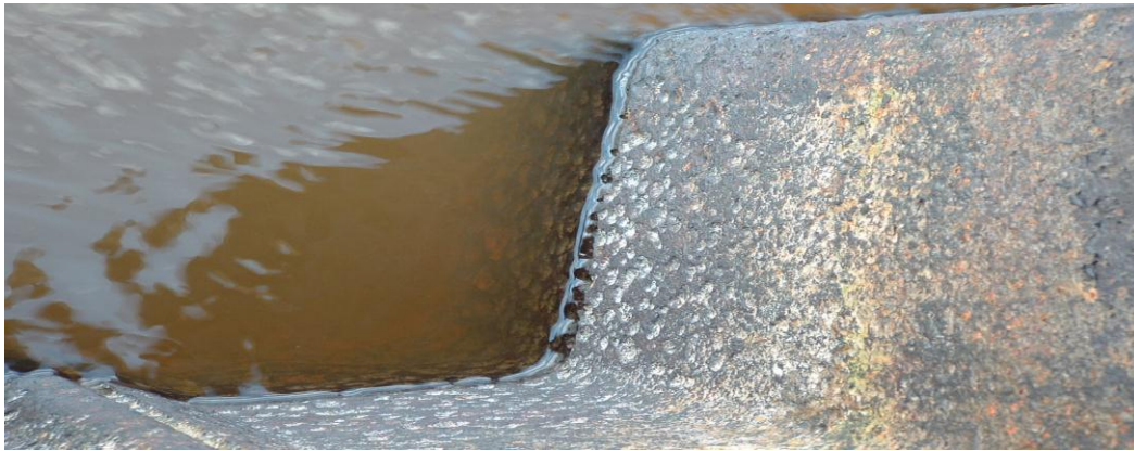
Photo 1. Bulkhead Pitting at Superior Entry
